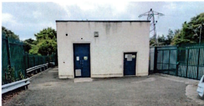
Figure 2 – Existing Malahide Substation.
